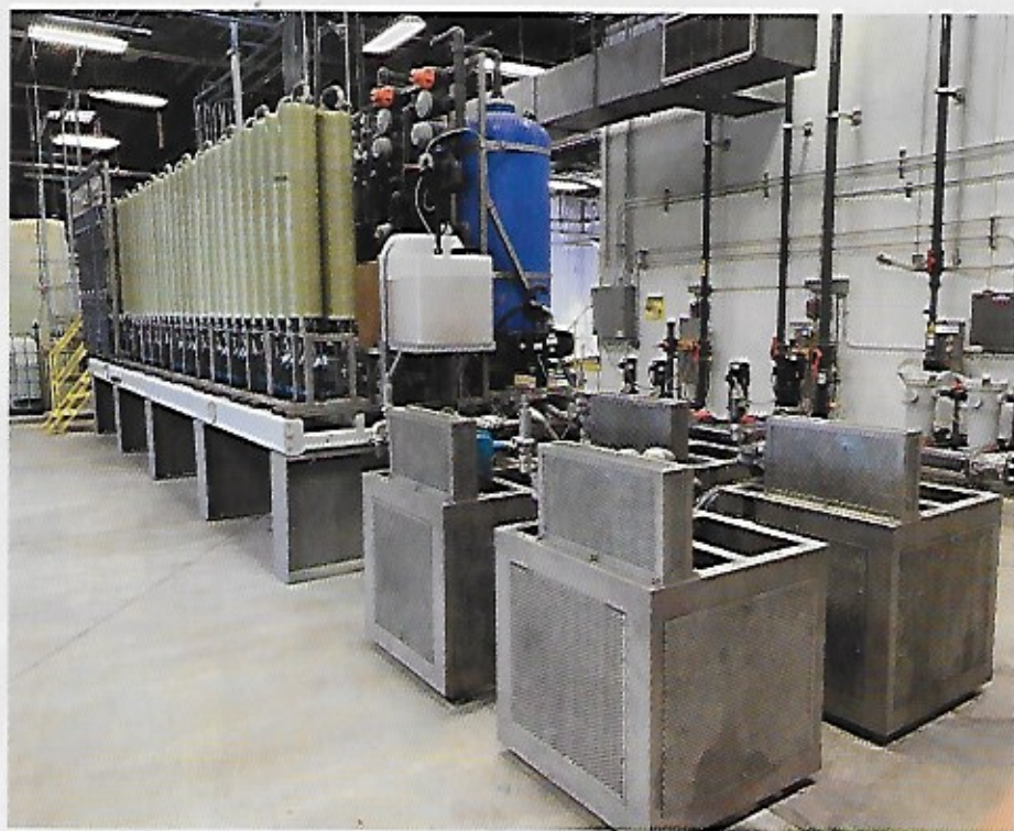
100,000-gpd two-pass RO leachate treatment system
