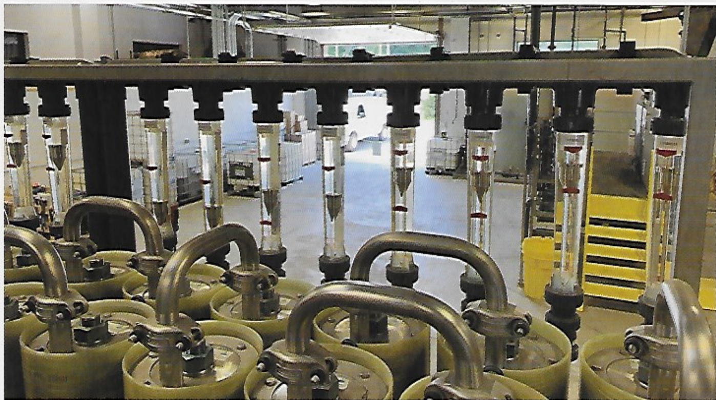
Leachate treatment effluent flowmeters
