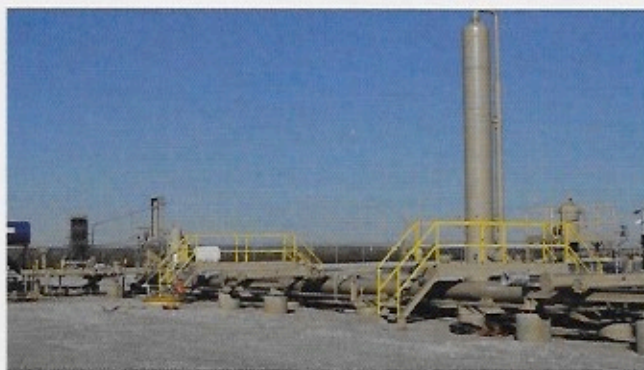
Figure 4. Pigging can help manage risks and operational costs that come from liquids blocking pipelines. Photo courtesy of WeldFit Energy Group.
